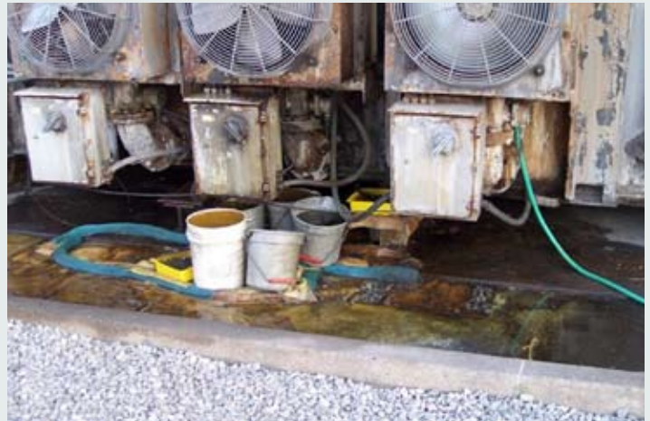
State of the transmission system, provided by ITC Holdings Corp.
