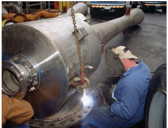
A welder modifies newly designed jets that spray steam into the condensers at The Geysers geothermal power plant. With a 750-megawatt output from 14 units, The Geysers is the largest producer of geothermal power in the world.
